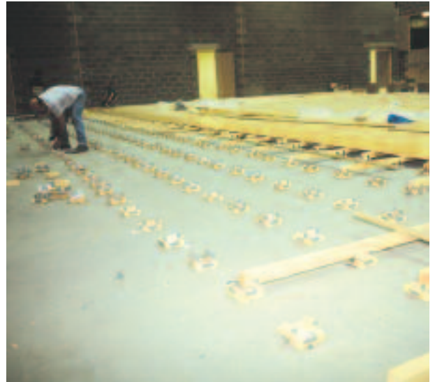
Playing surfaces in a sports hall must conform to BS:EN14904. A sprung or semi-sprung sports floor might typically be specified.
