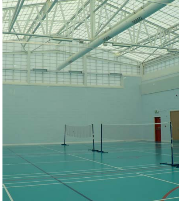
Jock Stein Centre in Hamilton, heated by gas radiant pipes.
